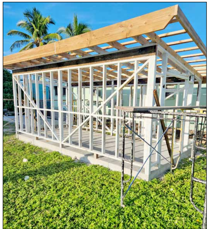
Construction of one of the water station buildings at Majuro Cooperative School.
